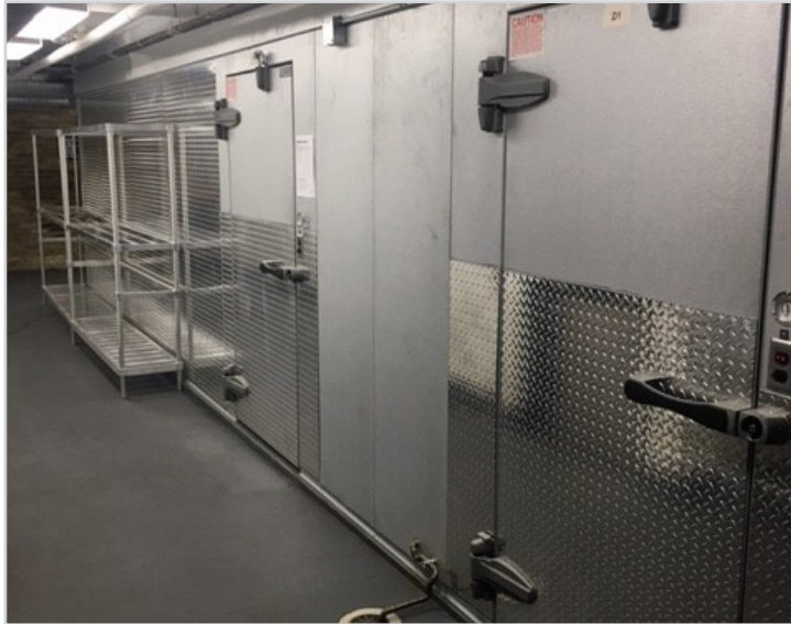
Walk In Coolers Downstairs
